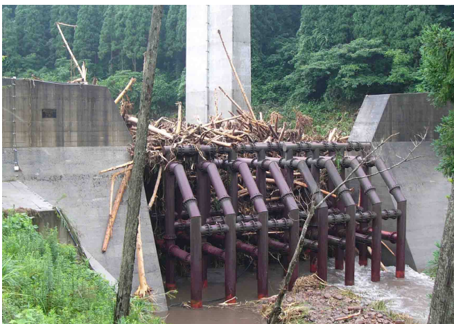
Photo 9 Capture of woody debris (Kitazato river dam)
